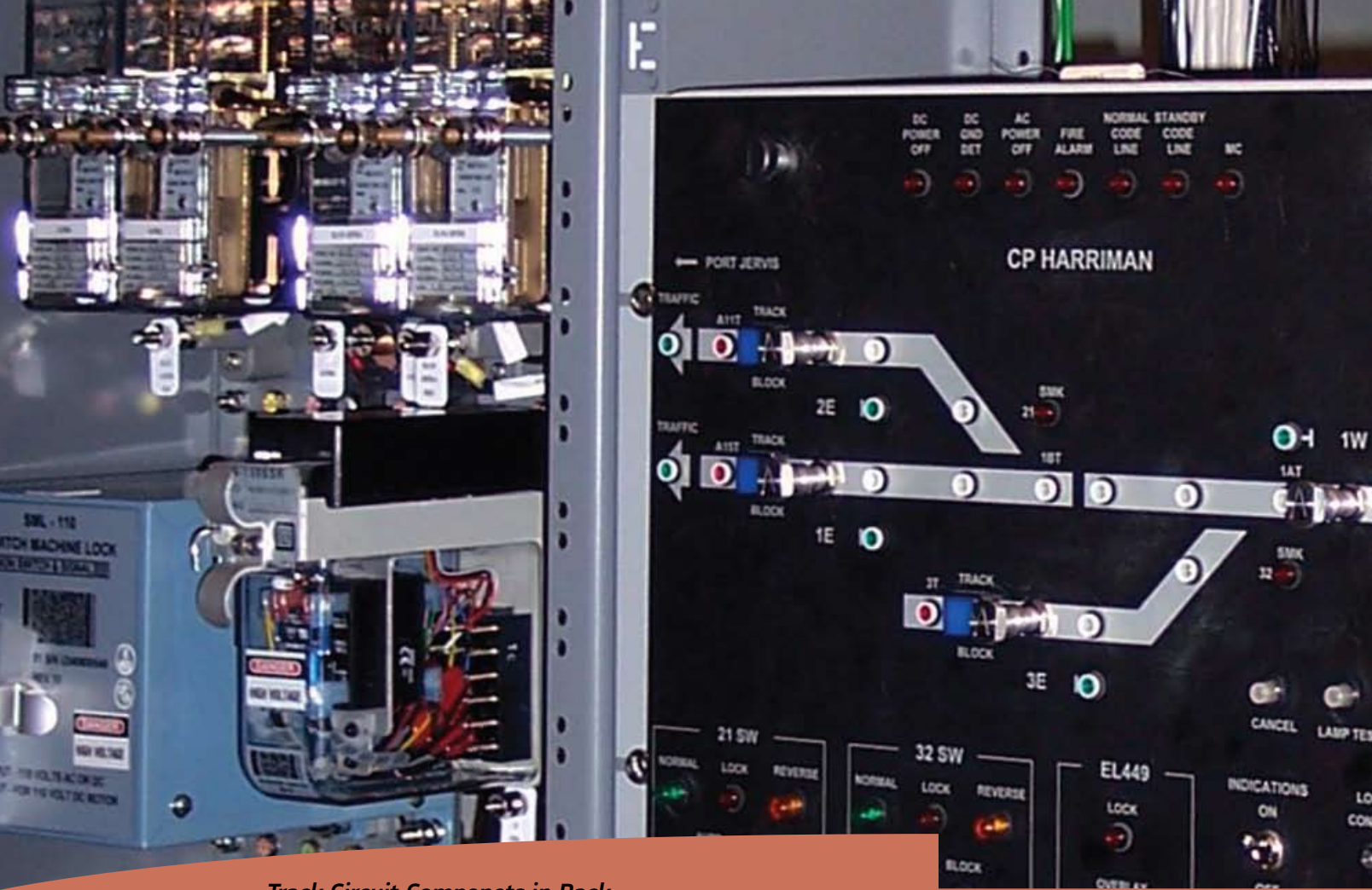
Track Circuit Components in Rack
