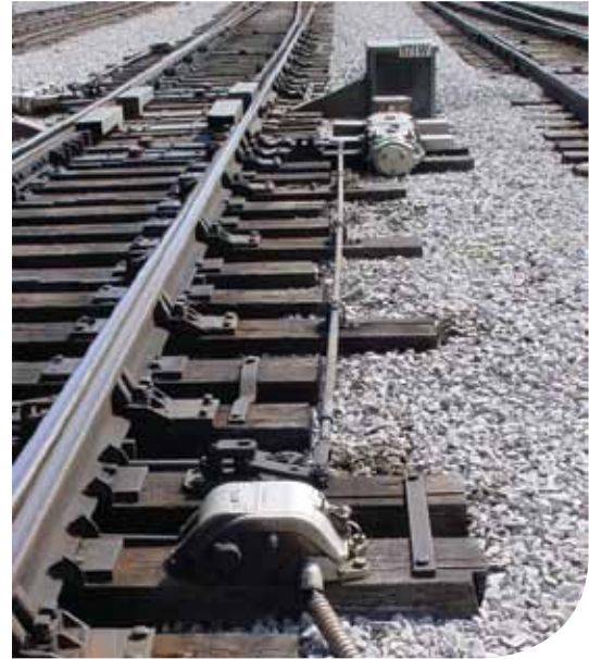
Switch Circuit Controller installed at customer location
