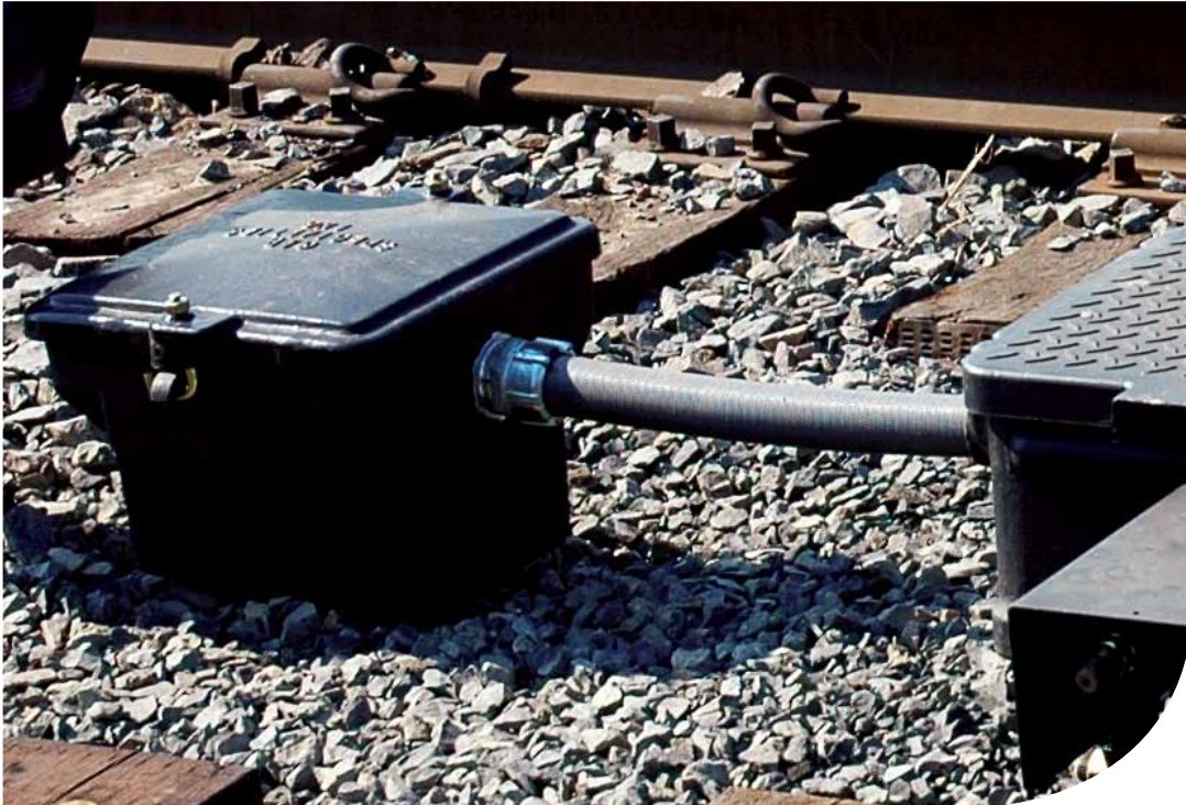
Junction Terminal Box installed at customer location
