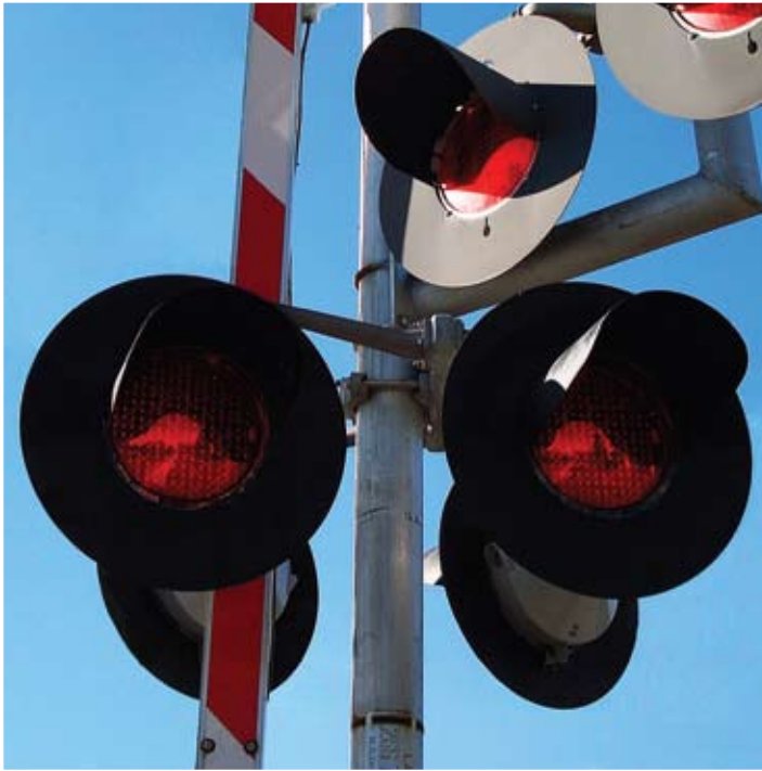
AURORA 12" LED Highway Crossing Retrofit
