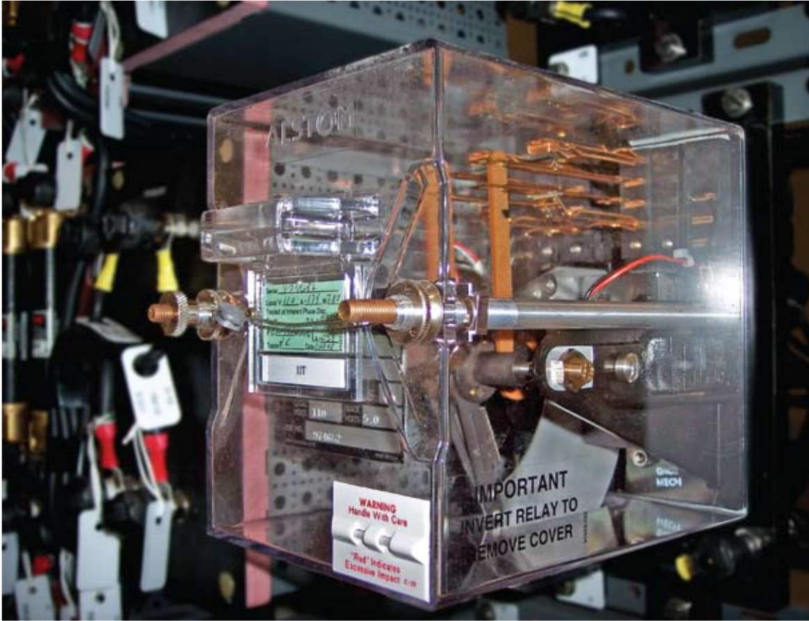
B2 Vane Relay Installed in Track Circuit Rack for customer.
