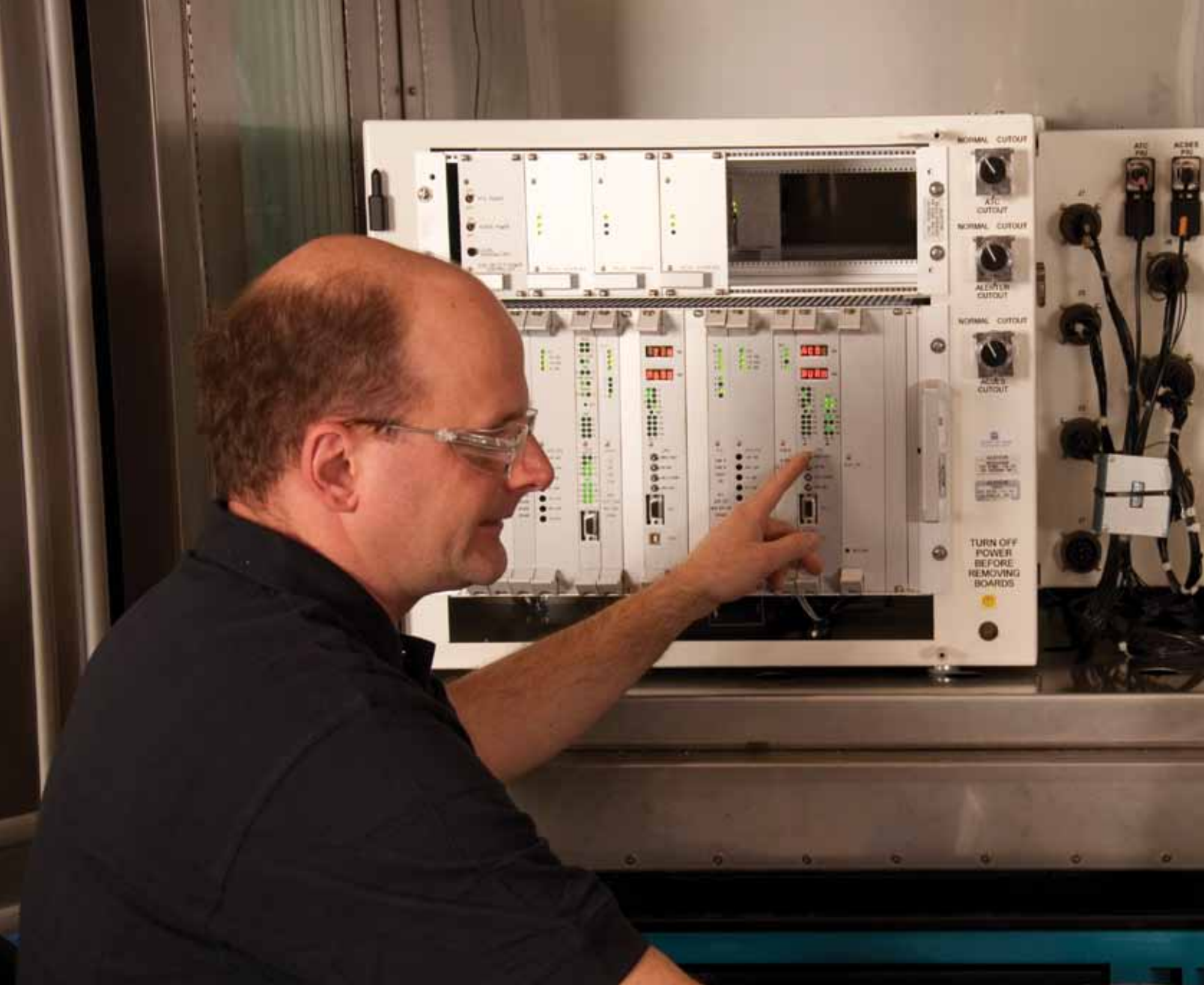
Testng of Microcabmatic III (ATC/PTC) at the Rochester Site © 2010 Alstom Transport
